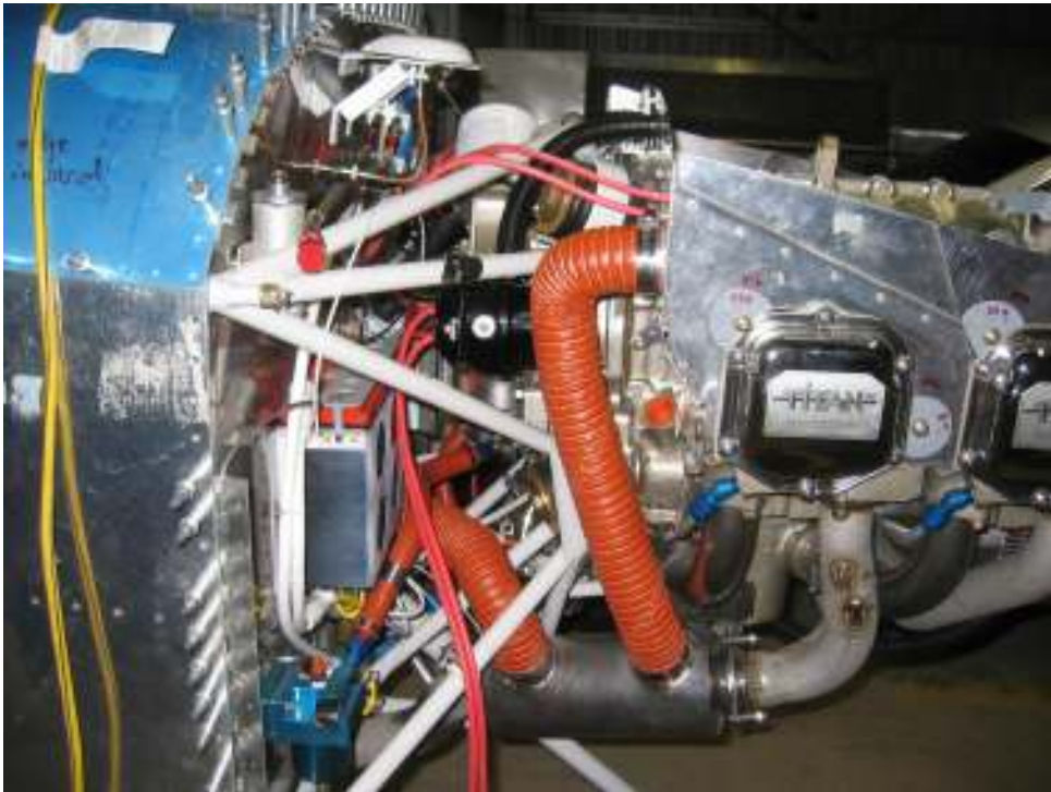
Install SCAT tube for cabin heat, adjust muffler positions, reroute fuel line Mount 2" flanges
