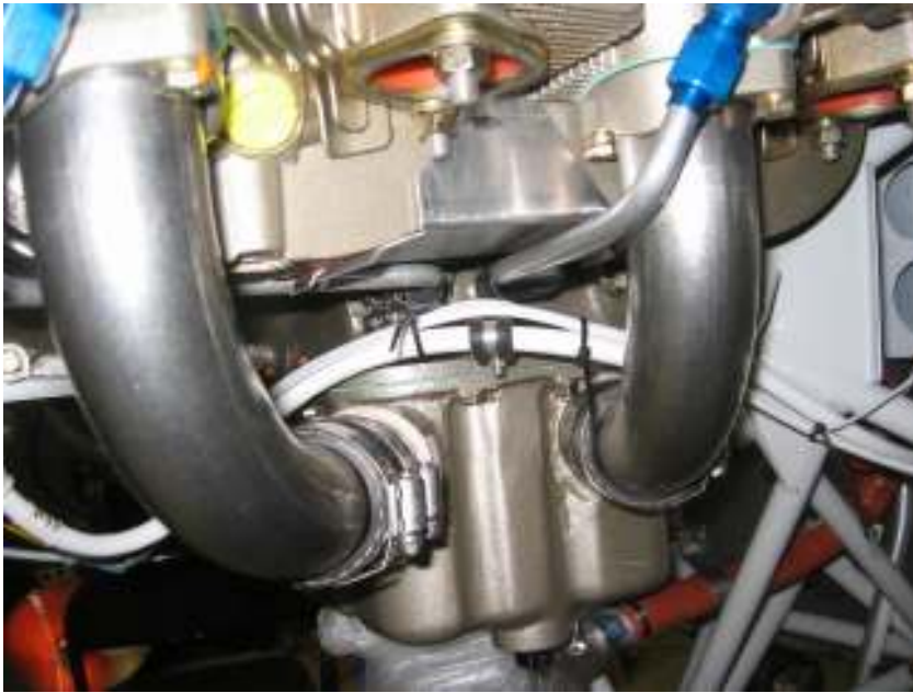
Bolt in adel clamp for starter cable
