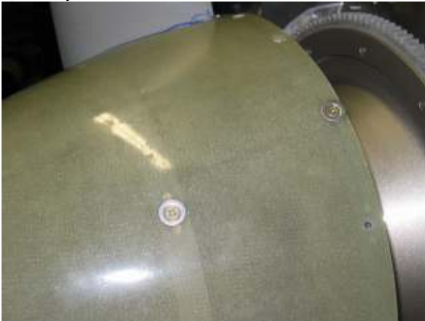
Install nutplates for spinner Install a few Adel clamps in the engine compartment Trim air inlet fairing further to fit airbox airseal material Trim left front baffle to fit the added glass clothe on the air inlet Total time: 5 hours (1040 hrs)
