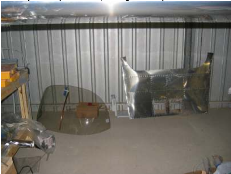
Rivet access panel supports, drill compass and COM 2 antenna hole, mount COM 2 antenna on windshield
