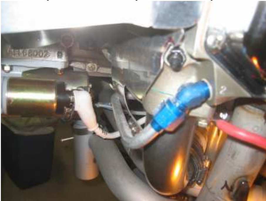
Mount prime connector (cut left baffle bottom to clear) Install heat shield for starter and alternator wires Total time: 5 hours (953 hrs)
