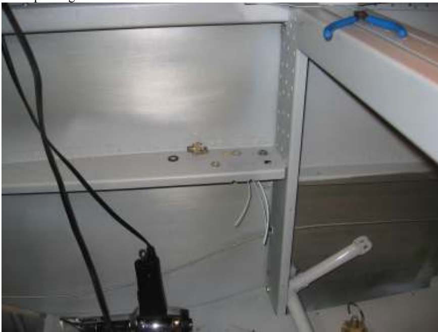
Running pilot and co-pilot phone and mic wires to the rear of arm rest. Total time: 7 hours (686 hrs)
