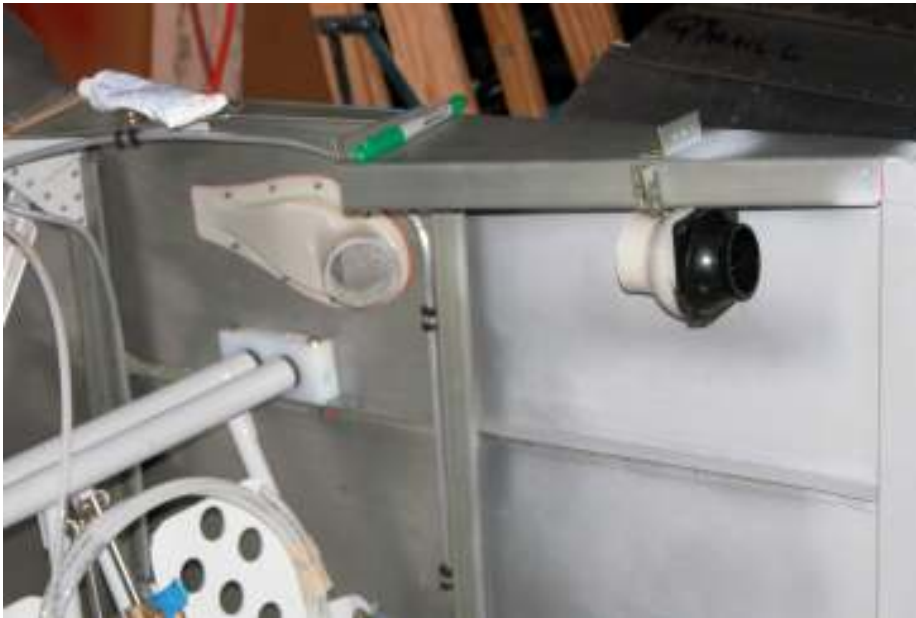
RTV right NACA fresh air inlet and mount air vents
