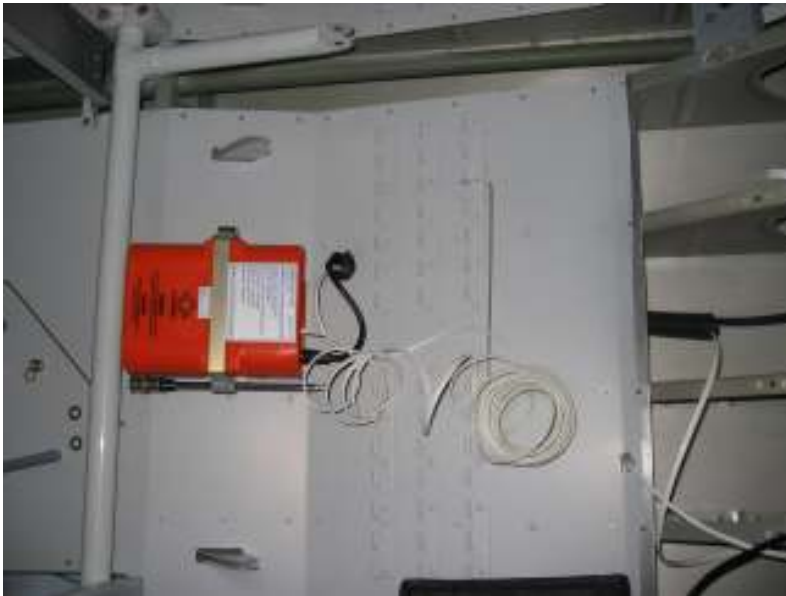
Mount ELT and drive hole for conduit Drill and rivet ends for the aileron push rods
