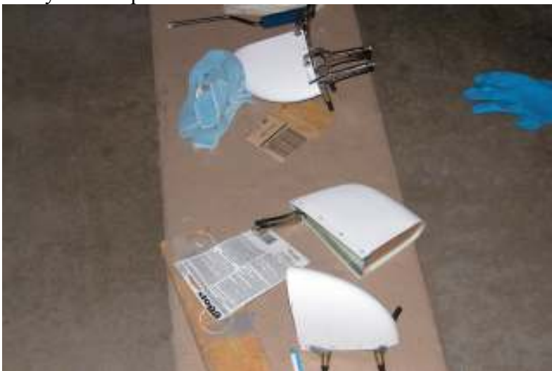
Drill, countersink, glue aluminum strip for HS and VS tips, make pattern for VS tip closure
