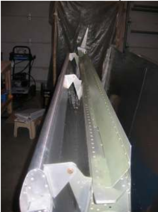
Fit both flaps to wings, insert bushing Remove rudder Clean up fuselage and begin preparation for interior painting Total time: 5 hours (269 hrs)
