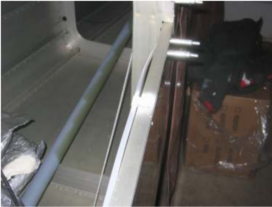
Fabricate and install two clips for static line Total time: 5 hours (264 hrs)
