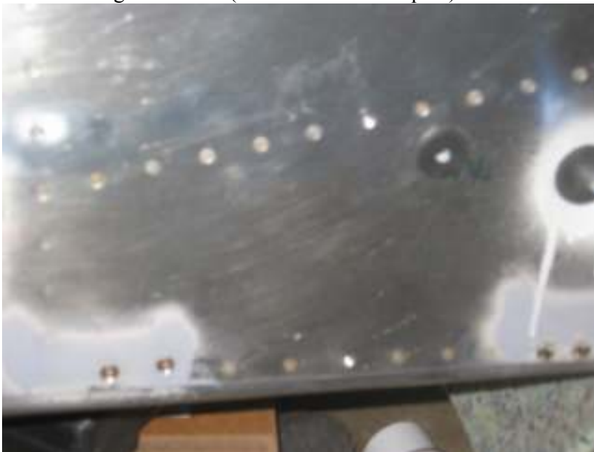
Counter sink two screw holes on the skin for each gear mount Finished fuel line through gear mount Drill holes for vent tube on the column Partially completed vent line on the right hand side
